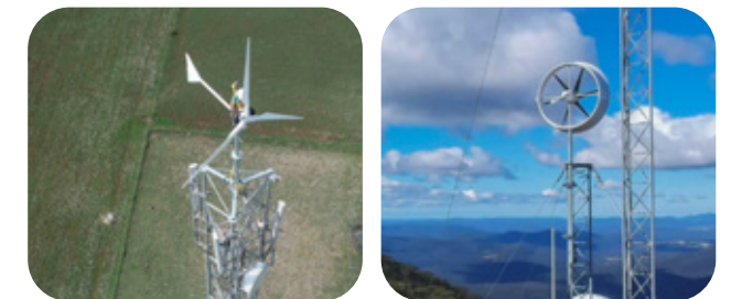
Figure 3: Telecom base station with wind turbine technology (Revayu Energy) (left) and (Diffuse Energy)(right)
